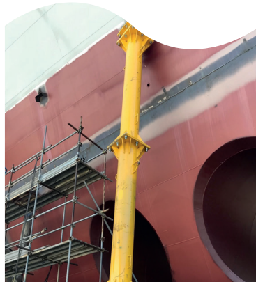
Carpentry, welding and finishing work for the assembly of semi-finished products, blocks or composite elements (sections) of hull
